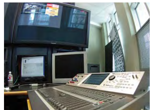
Canwest Control Room
