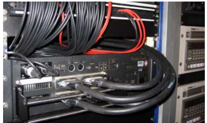
S-4000H in control room (Babel 2008)
