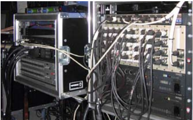
S-4000S, S-4000H and S-4000SP installed in studio (Gente de Mente 2008)
